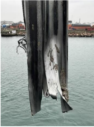
Figure 7 Damaged sheet pile toe as retrieved.
